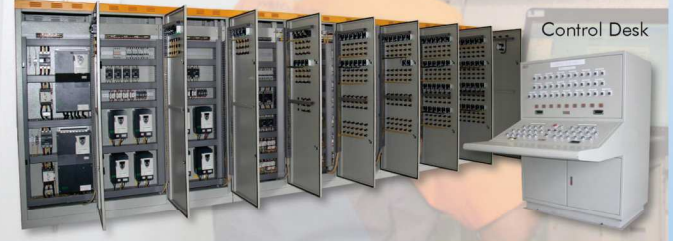
Fixed Type (LV MDB, MCC, Inverter, and Capacitor Bank Panel)
